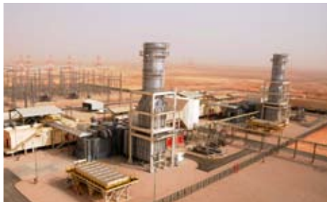
Amal Power Station EPC Project for PDO
