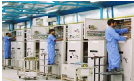
MV Switchboards Assembly Facility - Muscat
