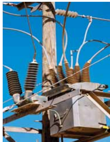
Auto Reclosers - PDO Project
