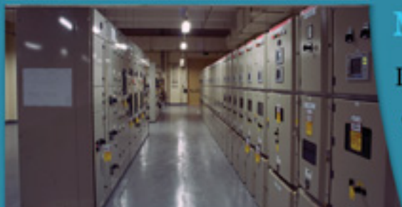
LV Switchgear Panels - Sohar Aromatics
