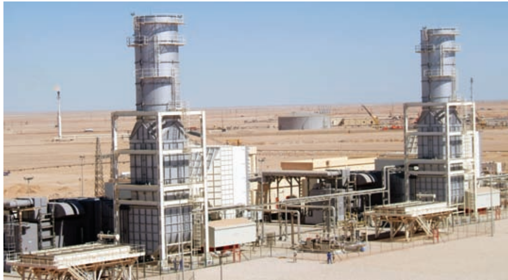
Mukhaizna Power Station for PDO
