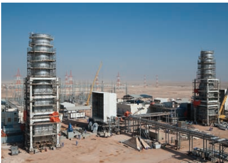
View of Amal Power Station Project for PDO
