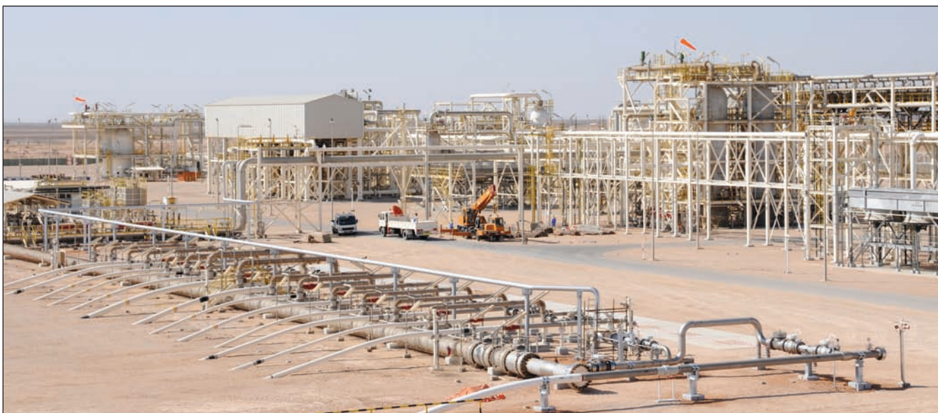
Burhan West DSS gas pipeline project for PDO was completed four months ahead of schedule
